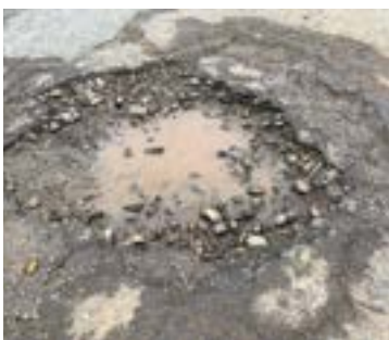
Let Martin and Sheila know about potholes you see in Gainsborough
